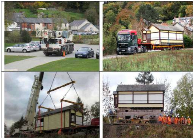
(L - R) 90 ton crane arrives, SB makes its way to site entrance, lift underway, SB on top of locking room
