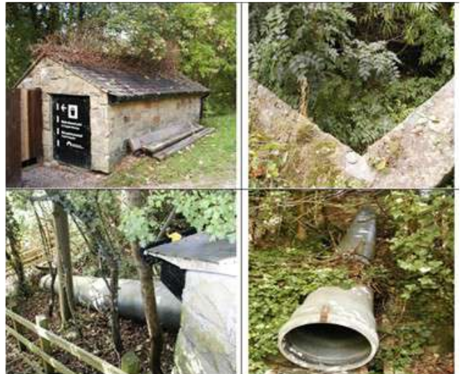
Remains of the Upper Dee Mills turbine power supply Clockwise from T/L - Sluice control from canal, remains of outfall to the river, looking up the turbine penstock, and down from sluice control shed
