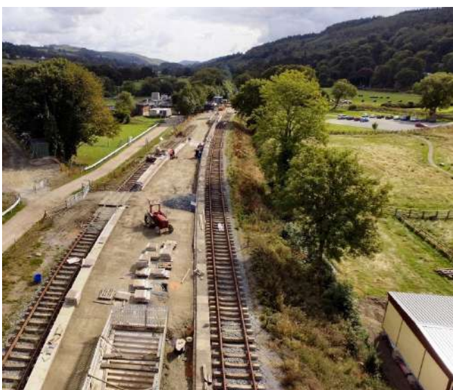
Looking east along the work site showing platform 1 & 2 walls Photo : Dewi Davies
