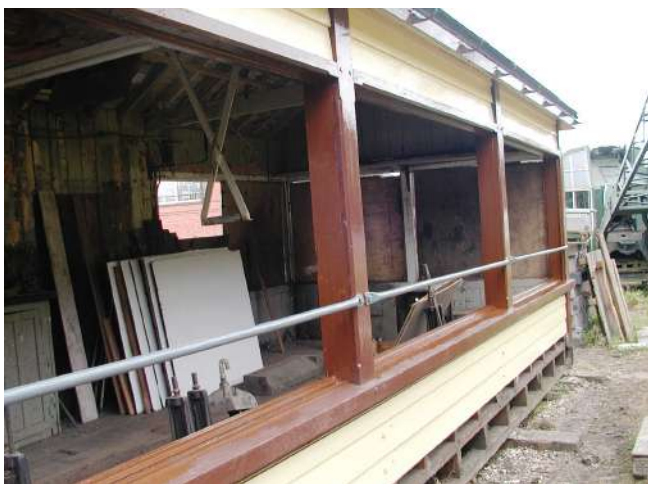
Front window frames under renovation now in chocolate and cream Photo : PR
