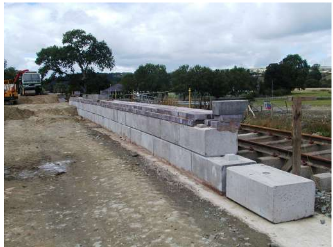
Platform 1 - Easi-blocs and second layer moving east - note infill – top left - also taking shape Photo : PR
