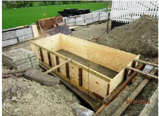
Shuttering at the west end to take the concrete bases for the canopy columns Photo: PM
