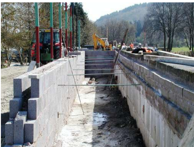
East end wall with tie bars and the beginnings of infill Photo: PR
