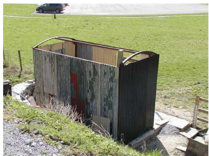
Almost complete - PH takes on real shape - roof next and then coat of black paint Photo: PR
