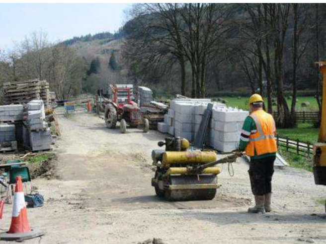
John Bearne compacting infill at Chicken Dock using the BOMAG roller Photo: GJ
