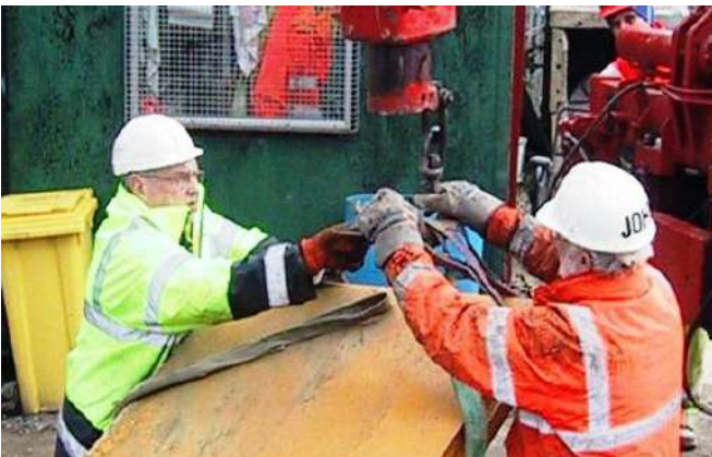
Doing what came naturally - Phil Carson (L) and John Heath prepare to hoist the cab of the mini-digger - Phil Morrey on crane duty Photo : PR
